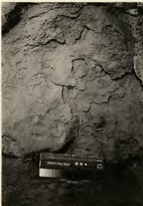
Fig. 23. Contour scaling and flaking of green sandstone 3' above grade at east wall of east transept (Photo: Anne Brackin).
